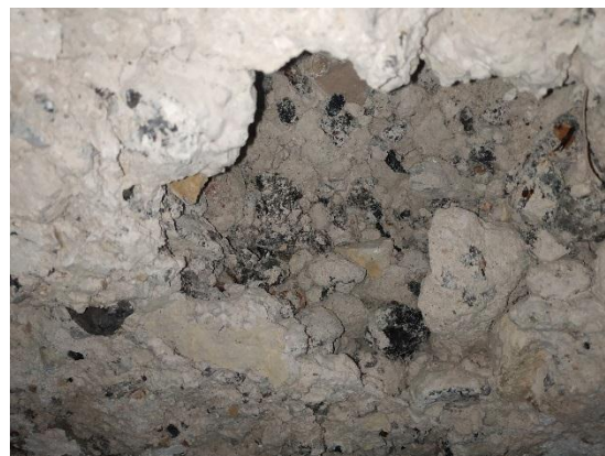
Image (9) shows Details of the location of the loss of concrete (the concrete sample that was studied)
