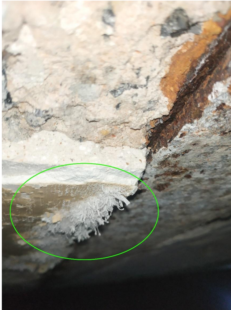
Image (7) shows render layers damage and the salts efflorescence on the color layer Surrounded by the green circle, the salt sample was taken from these salts efflorescence
