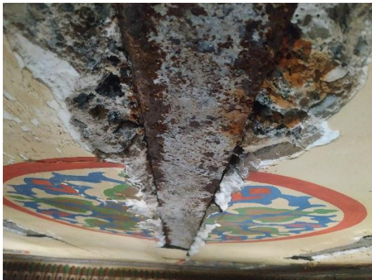
Image (5) shows The spread of rust in iron beams and roof concrete
