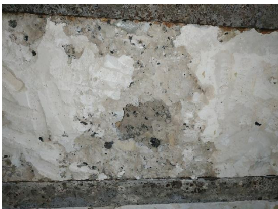
Image (8) shows Parts of concrete falling
