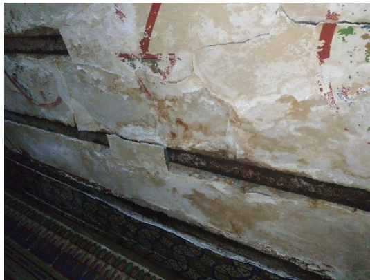
Image (6) shows peeling of colors, separation of render layers, and the spread of cracks
