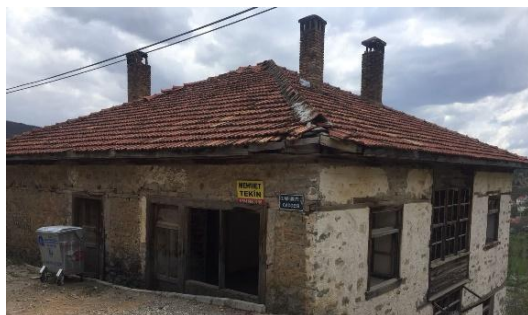
Figure 9: Butonned House roof sample [13]
